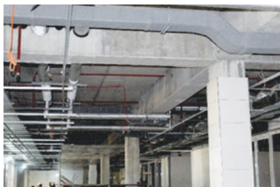
Cable trays and electrical installations
